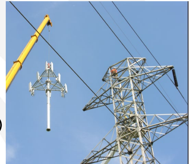
Collocation of a cell tower 14
