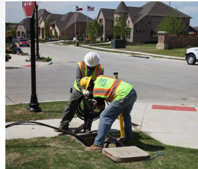
Handhole in a neighborhood
