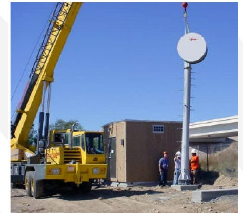
New microwave tower
